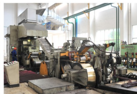
粗轧线 Rough Rolling Line
